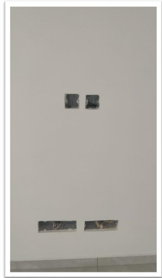
ELECTRICAL BOX FIXING
